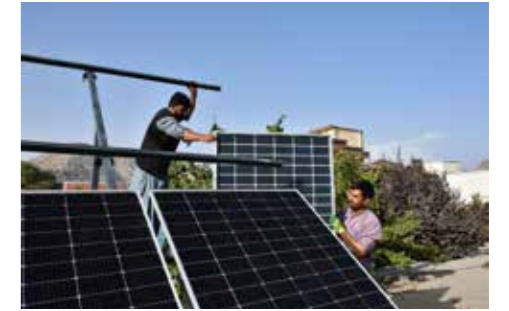
Sustainable NCA: With an average of 3085 hours of sunshine a year, solar is the obvious choice for electricity at NCA's Kabul office. Photo: Abdul Maqsood Shakib/Norwegian Church Aid, Afghanistan
